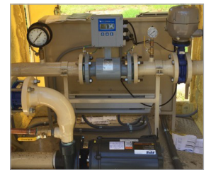
Pump and water meter, separated by a partition to protect electronics from water.
